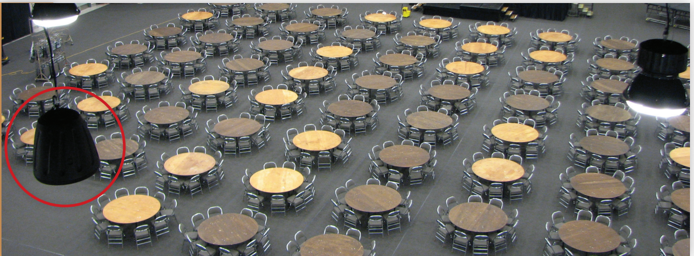
ONE OF 48 SOUND TUBE CEILING SPEAKERS INTEGRATED INTO THE VOCIA SYSTEM.
